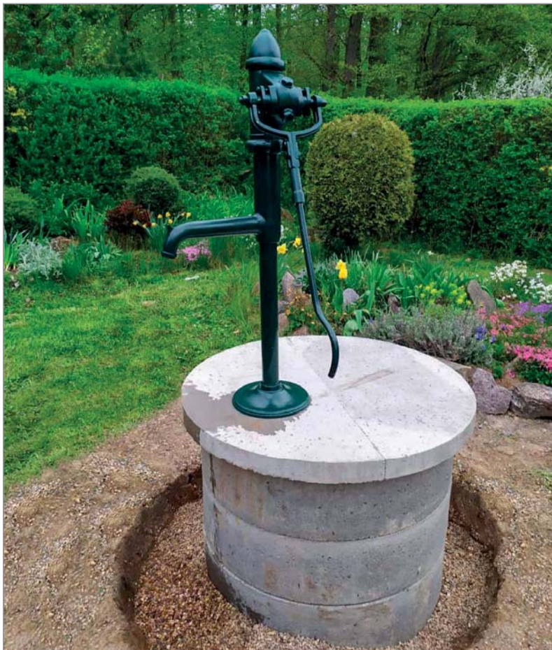
Demonstration of the realization of a new well with a standard T pump into the garden.
